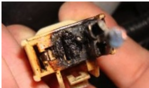
The result of a 12 Volt gremlin attack. The black charring is indicative of an arc.
