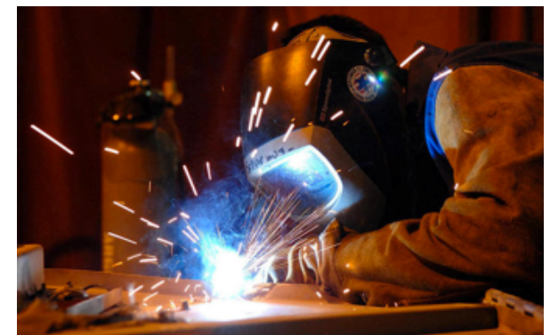
It’s just a bunch of electrons jumping from one location to another.
