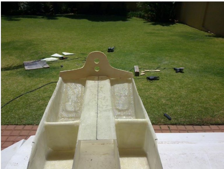
33. Looking from the tail end toward the front. The “jet intakes” can be seen in the molding. Temporary supports still in place.
